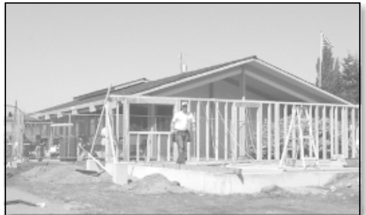
Work is progressing on construction of the new Cedarcrest Golf Course restaurant and relocation of the Pro Shop.
